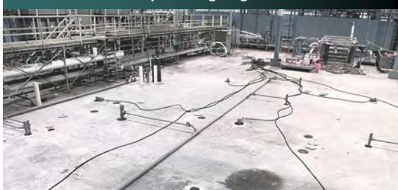
Thermal remediation system targeting sub-slab DNAPL
