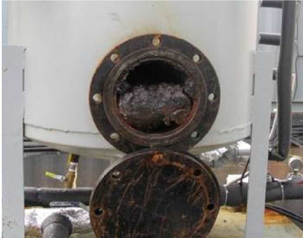
Figure 1: Heavy grease recovered through gas bubble floatation mechanism, Ft. Lewis, WA
