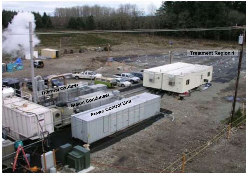
Figure 3: Layout of ERH treatment area, Ft. Lewis, WA
